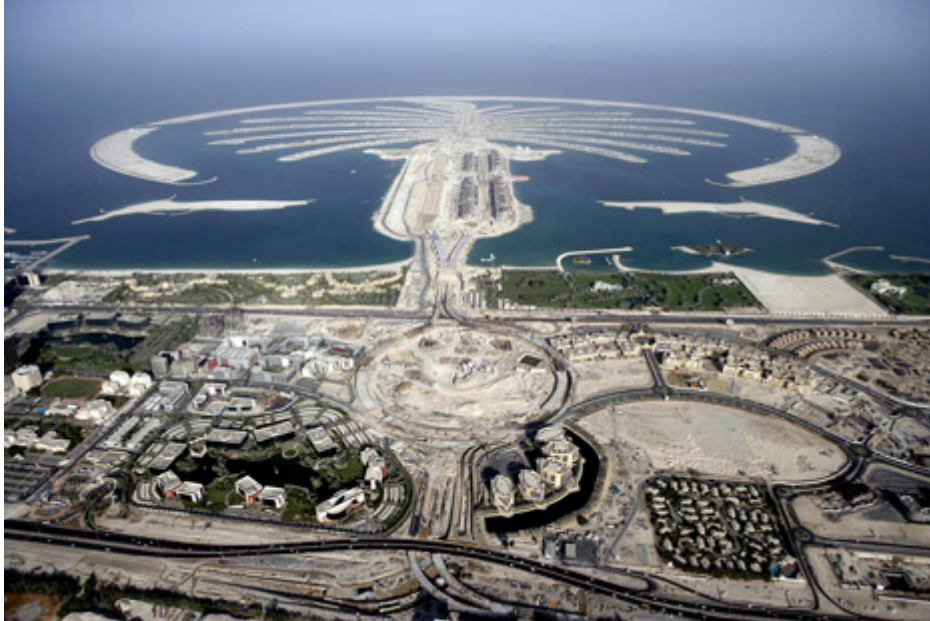
Aerial shot of The Palm with interchange construction in the foreground, UAE courtesy of arabianEye.com
